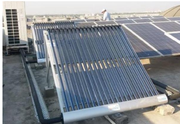
VRV without Solar heating system
